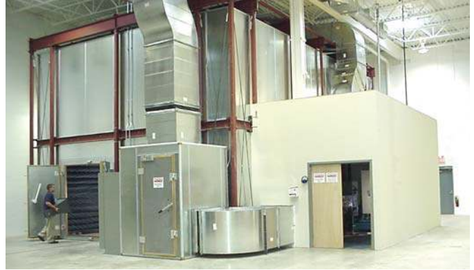
Large test chamber with auxiliary cooled shield room and noise controlled annex.
