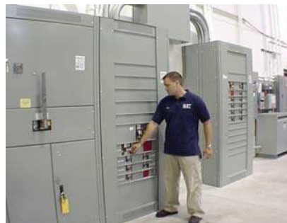
AC power entry at D.L.S. facility
